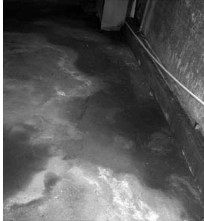
The basement of the Castle has a chronic moisture problem. The dampness has contributed to an infestation of mold that threatens many artifacts. Photo: Alexandra Allardt
